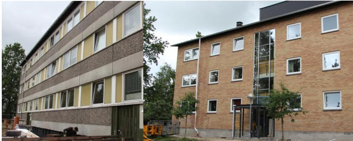
2 of the 3 blocks at Traneparken. The one on the left not yet renovated – the other after renovation.
