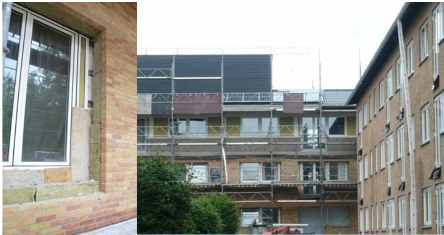
Figure: 190 mm insulation plus exterior solid standard bricks. Energy windows – aluminium – wood, 3-layer energy glass. In the panel walls: 285 mm insulation plus exterior solid standard bricks.
